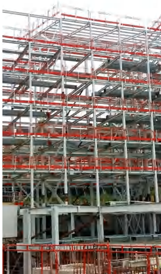
STEEL STRUCTURE EDGE PROTECTION SYSTEMS
