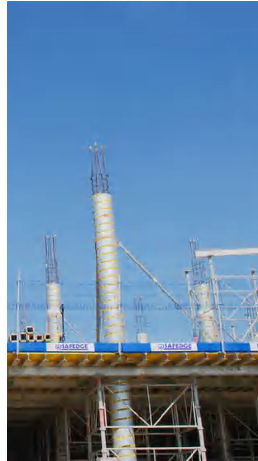
FORMWORK EDGE PROTECTION SYSTEMS
